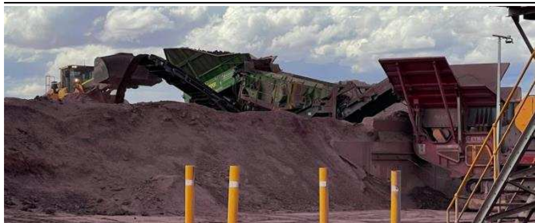
Figure 8: A dozer loads the scalper (green), which feeds the mobile crusher (red)
